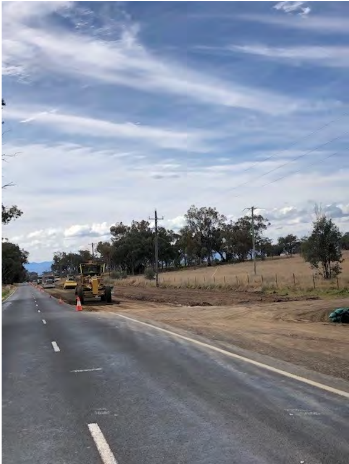
Plate 8 – Construction of an overtaking lane on Werris Creek Road for southbound traffic
